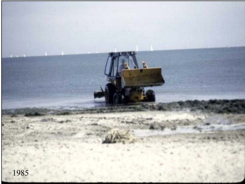
Front end loader used to push the algae to shore, where it is then piled up for later removal after some dewatering.
