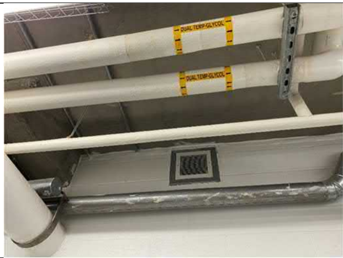
Dual Temp Glycol Piping
